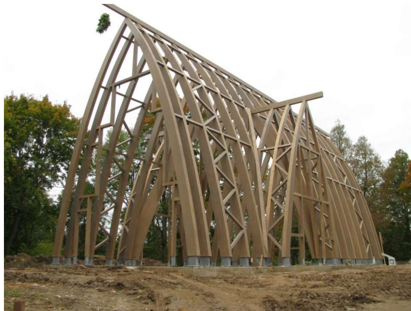
Fig. 3.9. The load bearing glulam structure of the church in Dubingiai
